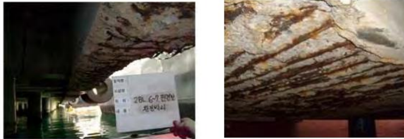
Fig 1 Corrosion problems of concrete structures
